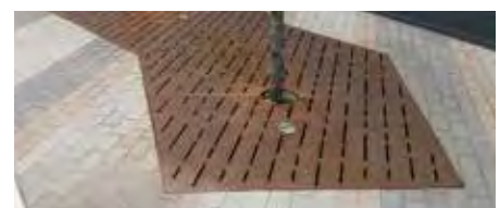
Tree trench filters are tree planting areas that include large underground areas with materials that store and filter stormwater
