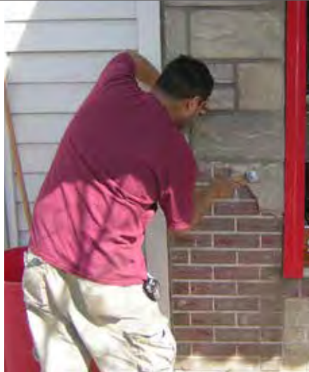
Repair deteriorated primary building materials.
