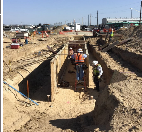
Formwork for Stormwater Planter west side of Brighton, south of 48th and Brighton intersection
